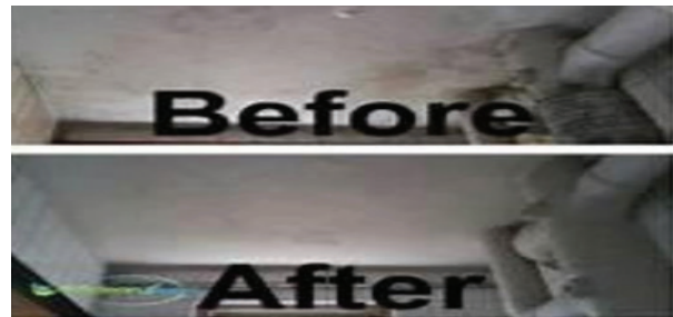
Fig. 5: Before and After
